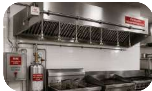
KITCHEN HOOD SYSTEM
